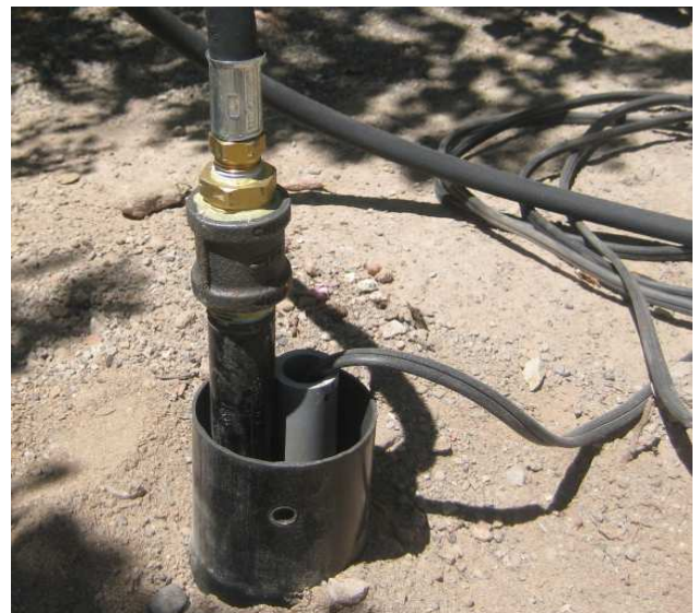
½” Coupling with brass ½” to ¼” reducer bushing and gas hose installed
